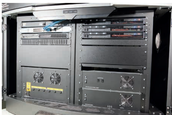
Fig 8. Electronics and laser control cabinet.
